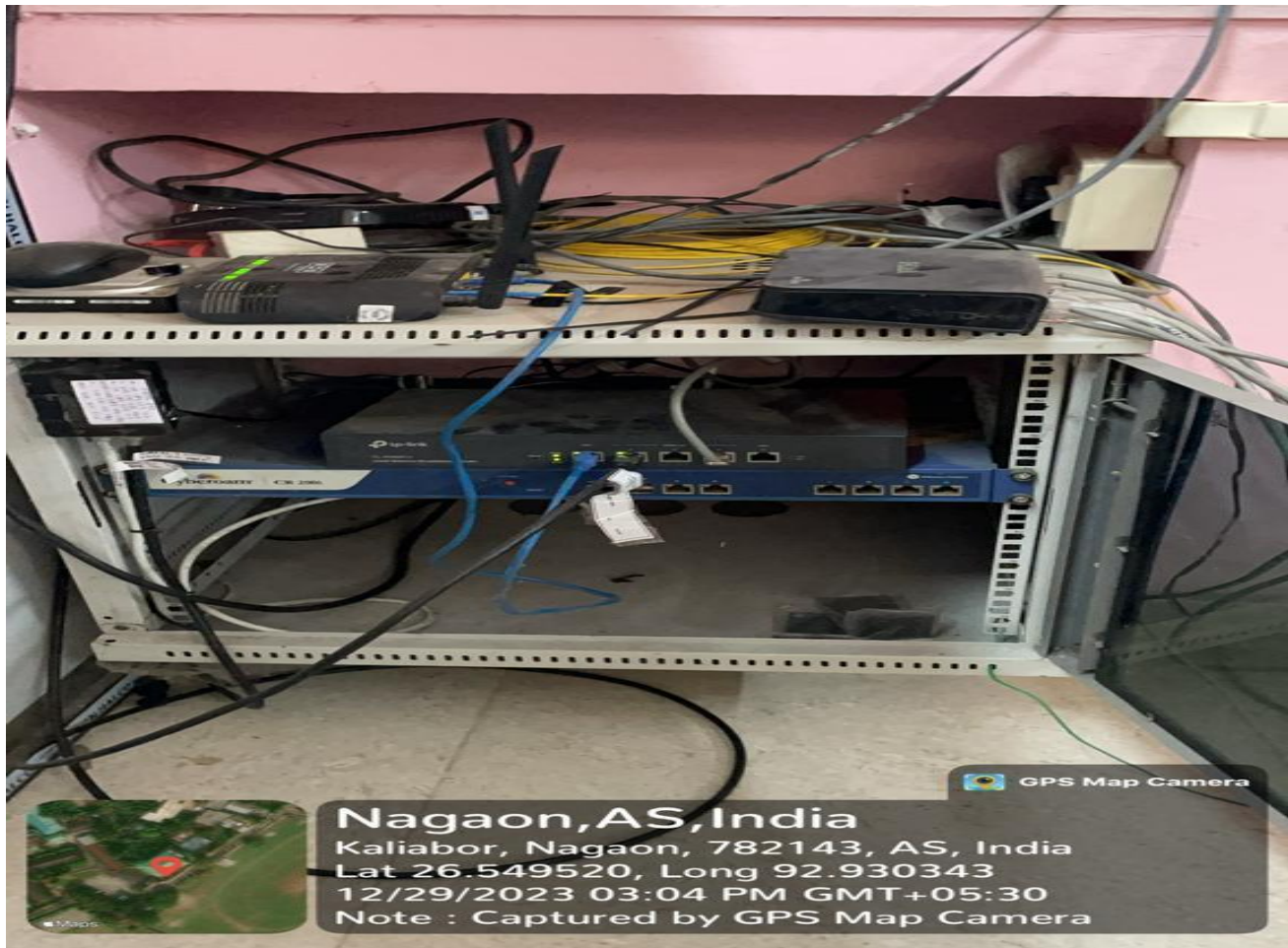
ROUTERS AND SWITCH
