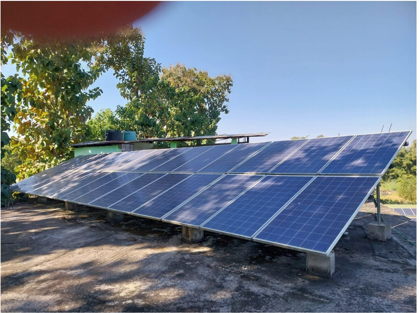
Shaded panels of the solar plant.
