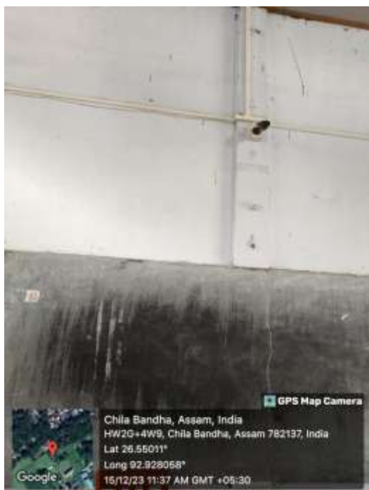
CCTV Camera inside class room
